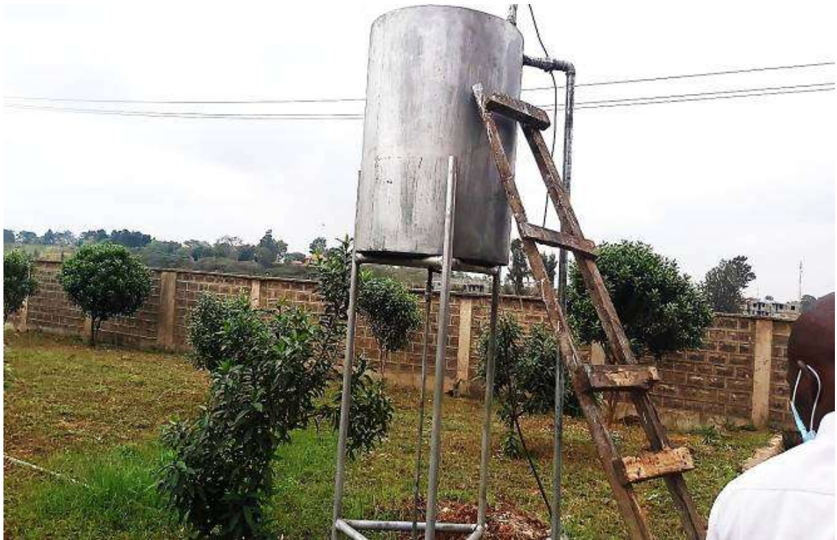
Figure 6: The raised 500litres diesel metallic tank outside the MWTI shelter (Source: field work)
