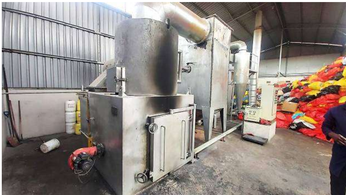
Figure 8: The installed MWTI (Source: fieldwork)
