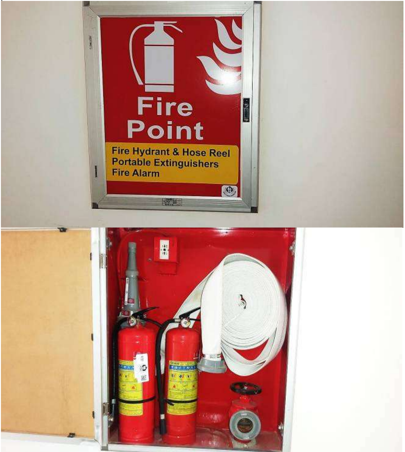
Figure 18: One of the well-marked fire management points within the hospital premises (Source: Field work)
