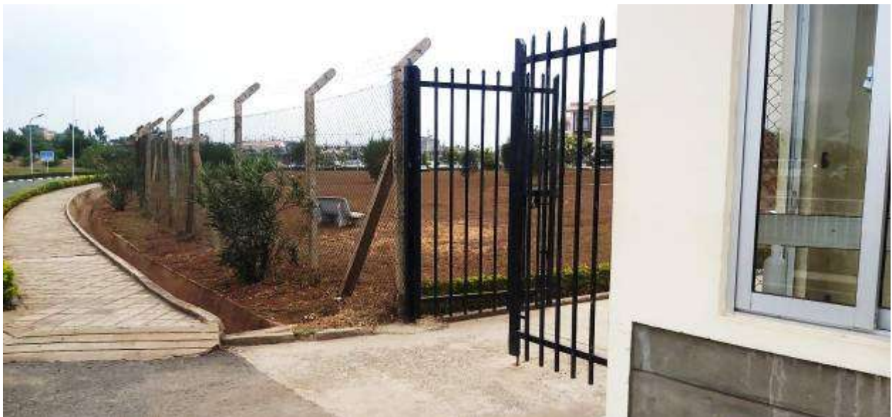
Figure 3: The chain-link fence around the two wards identified for renovation (Source: field work)
