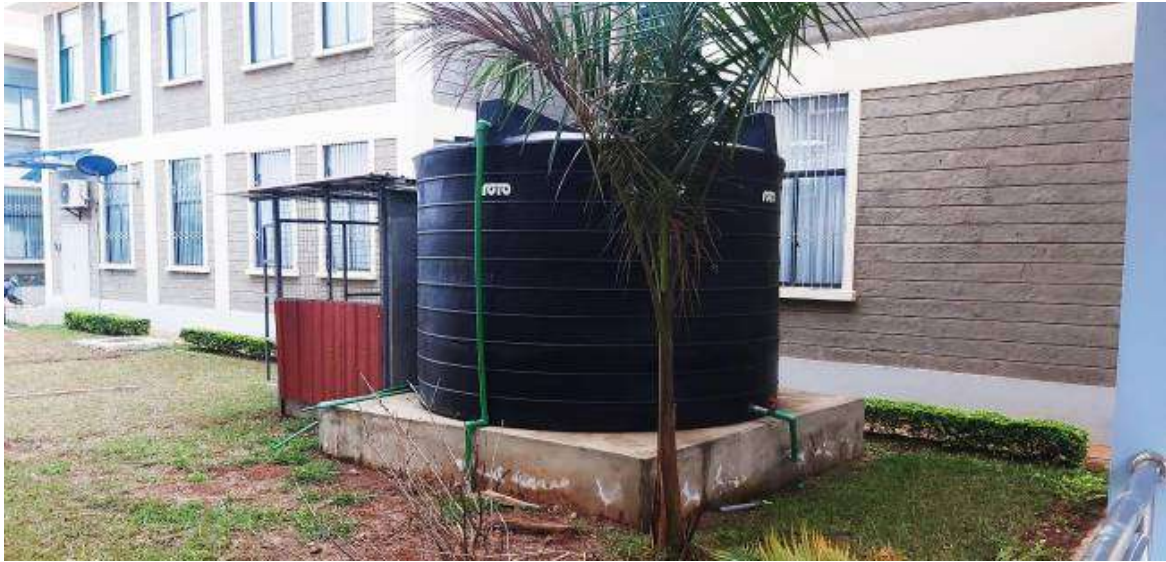
Figure 16: One of the surface water storage tanks within the hospital (Source: Field work)
